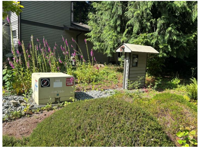
Photo 37: Typical BC hydro pad transformer and meter for septic pumps and streetlights.
