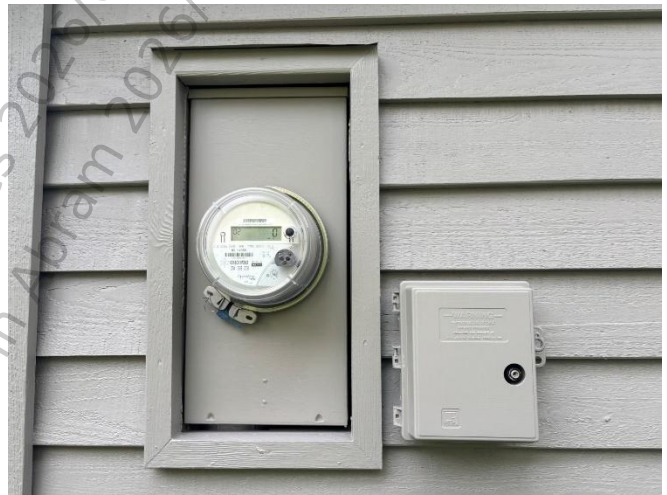
Photo 38: Typical meter for a townhouse unit.
