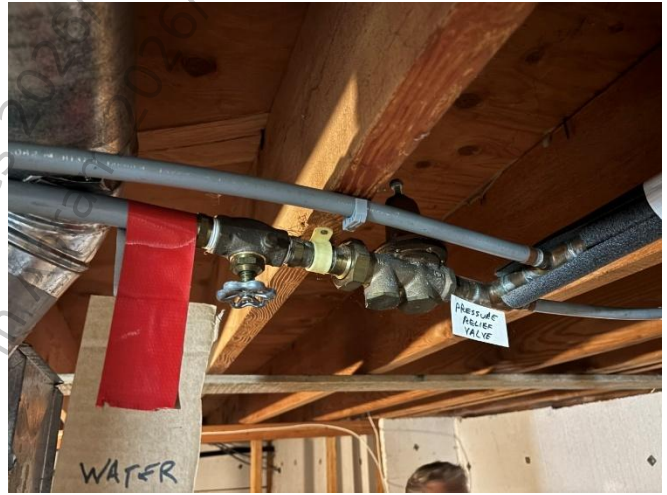
Photo 33: Water shutoff inside a unit.
