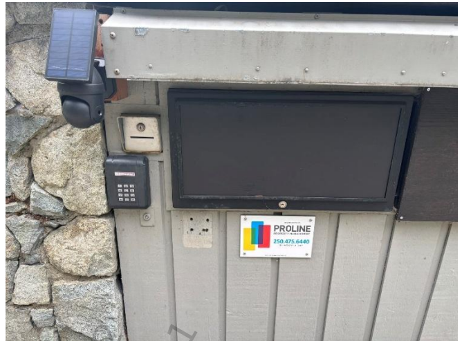
Photo 45: Enterphone and keypad at main entrance to complex.
