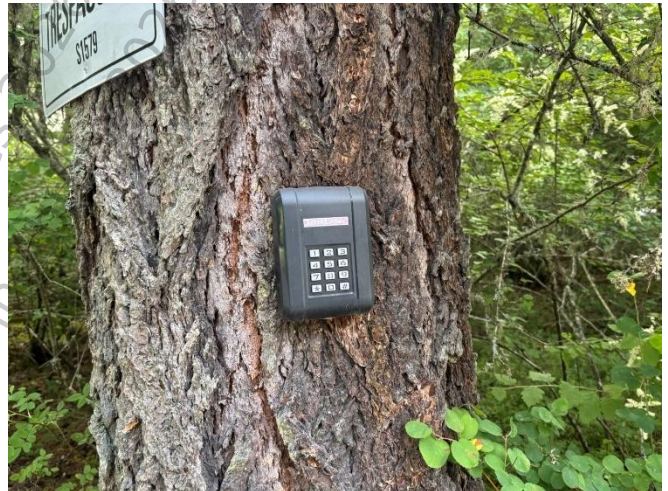
Photo 46: Keypad providing access to RV storage lot.
