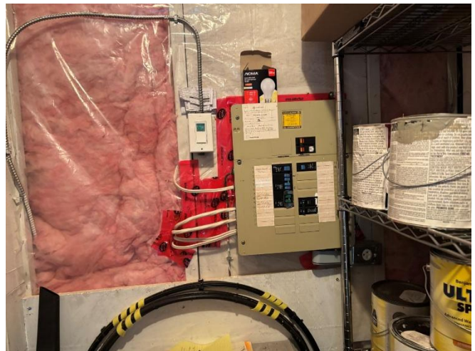
Photo 39: Electrical panel inside utility shed.
