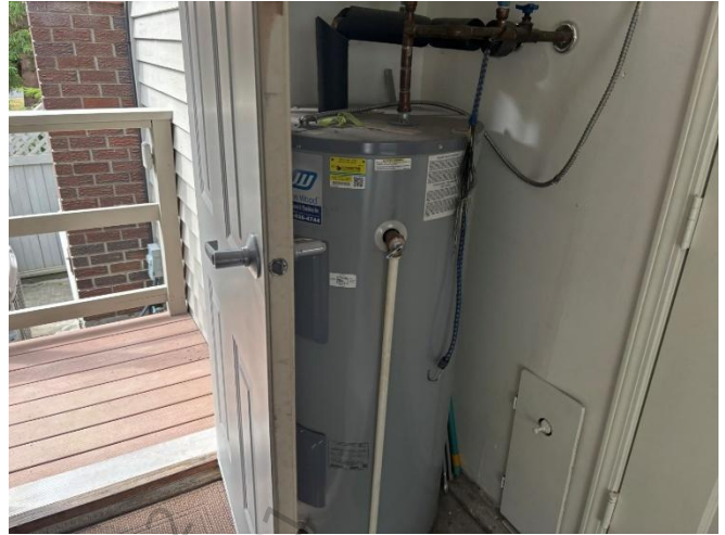
Photo 31: Typical hot water heating tank.
