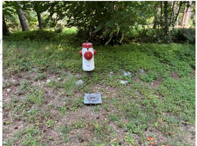
Photo 20: Typical fire hydrant.
