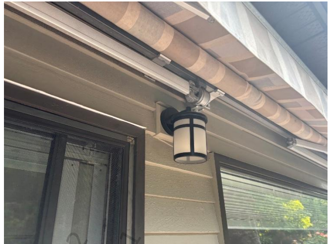
Photo 40: Typical wall-mounted light fixture at townhouse units.
