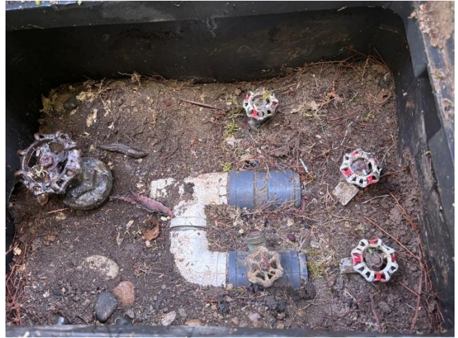
Photo 32: Water line splitting to supply domestic water to each unit within a pod.
