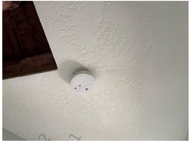
Photo 19: Typical townhouse unit smoke detector.
