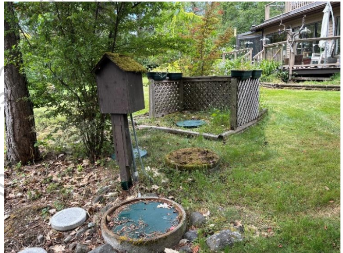
Photo 35: Typical septic tanks.
